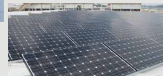
Photovoltaic facility at Ochang Plant
